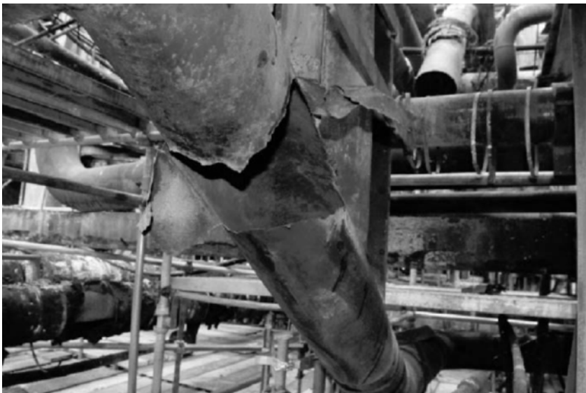
Figure 2.7. Rupture in 52-inch component of line, courtesy CSB.
