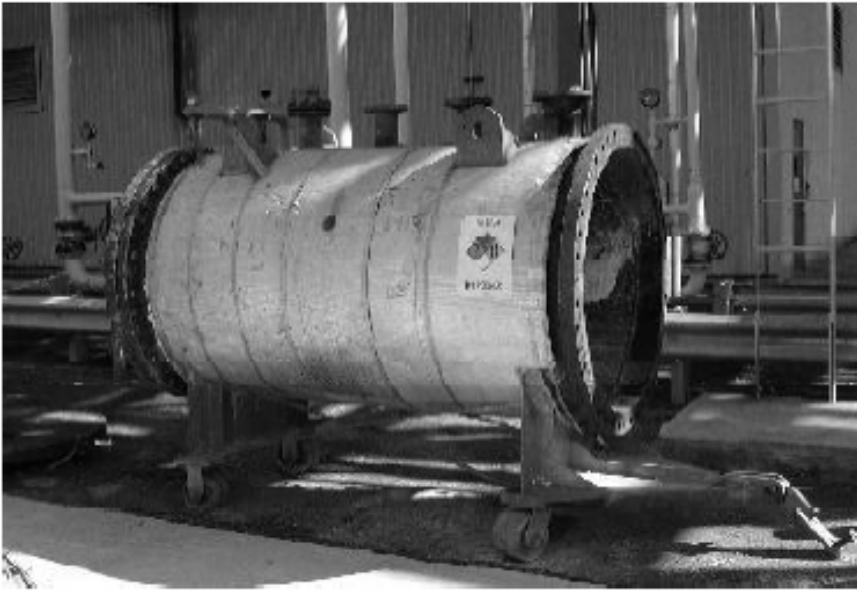
Figure 5.45. Polymer catch tank, Ref. 5.50.
