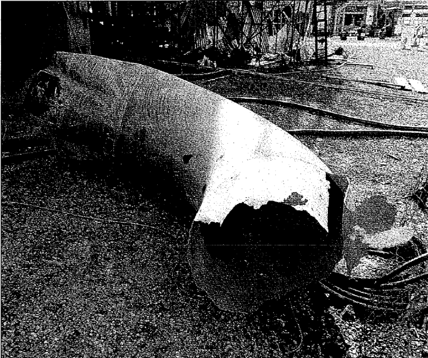
Figure 3.19. The 30 inch flare line elbow that failed and released 20 tons of vapor, source (HSE, 1994).
