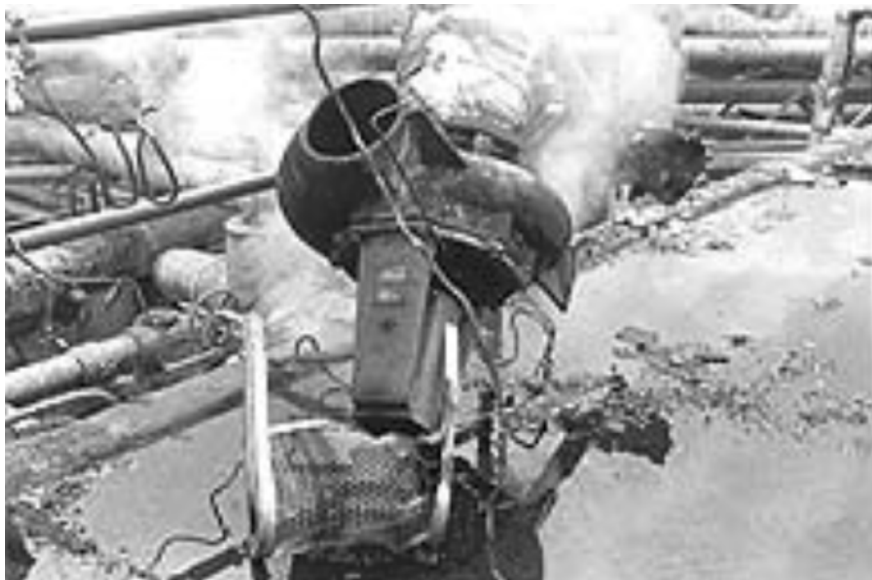
Figure 5.2. Pump explosion from running isolated.
