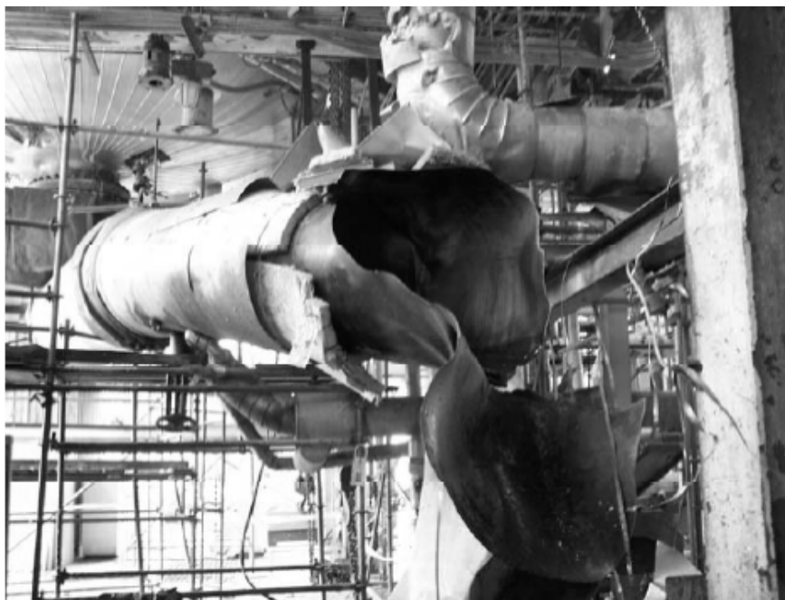
Figure 5.8. Ruptured pipe from reaction with heat transfer fluid.
